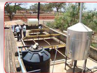
Solar Water Heating System Installed in Multi-end Silk Reeling Unit
