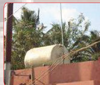
Ushma Shoshak on Boiler Chimney and Insulated Tank
