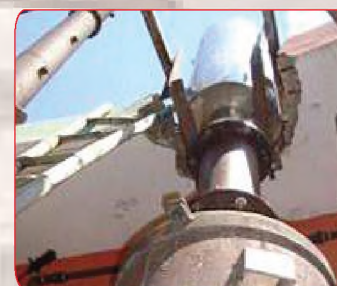
Ushma Shoshak Unit Mounted on Boiler
